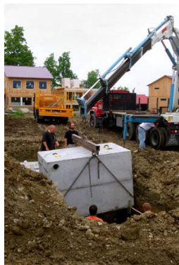
Buried cistern, Ithaca has the capacity to collect 30,000 gal of water.
