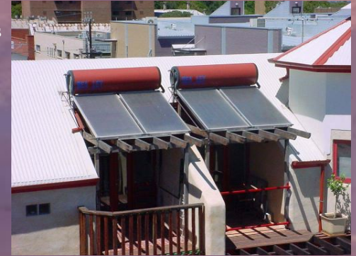
Solar Hot Water Panels (Photograph provided by Ecopolis Architects)
